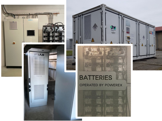
BATTERY STORAGE ASSETS - LI-ION AND REDOX FLOW
