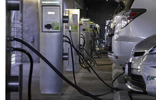
EV CHARGING INFRASTRUCTURE
